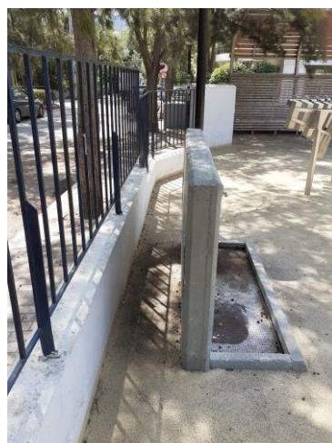
Figure 7.7: Space behind the water taps
